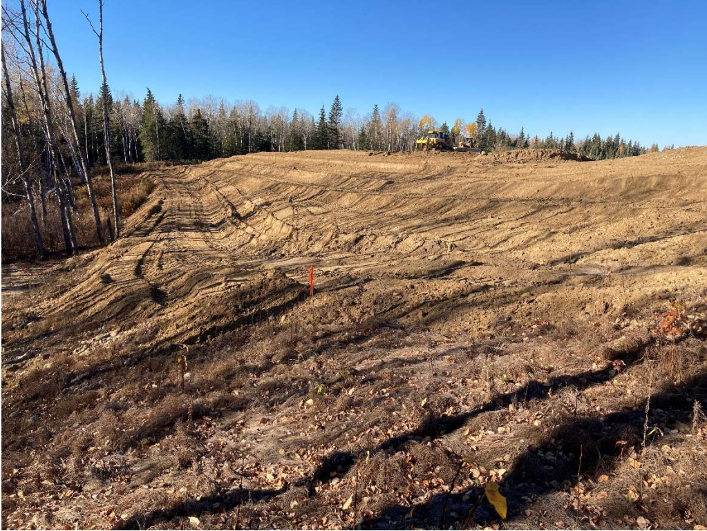
Photo 5: Photo taken looking southwest of the interim remediation of the erosion on the back of the south slopes.
