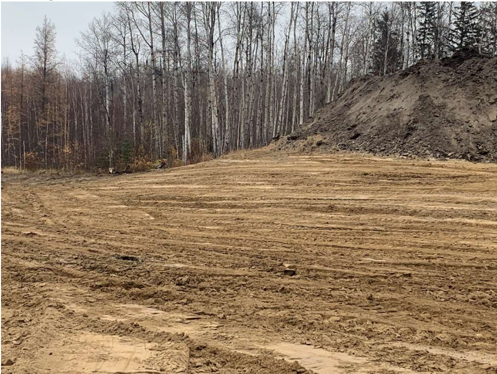
Photo 2: Photo taken looking North of the topsoil salvaged from the low lying area.
